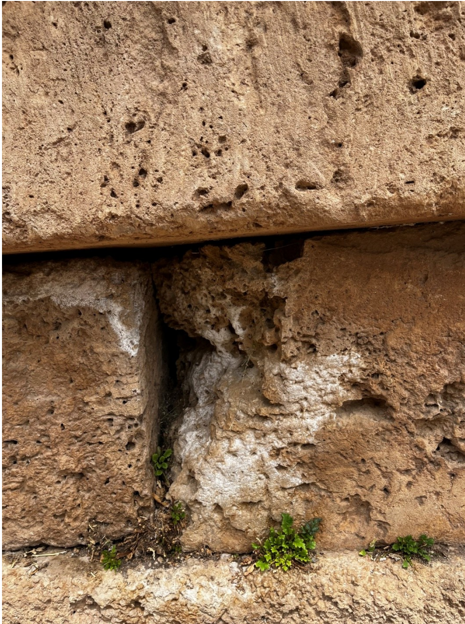
Figure 6. Localised weathering and material loss on a stone element of the Temple of Apollo. The photograph illustrates the development of a porous surface texture and the deterioration of the stone's superficial layer.
