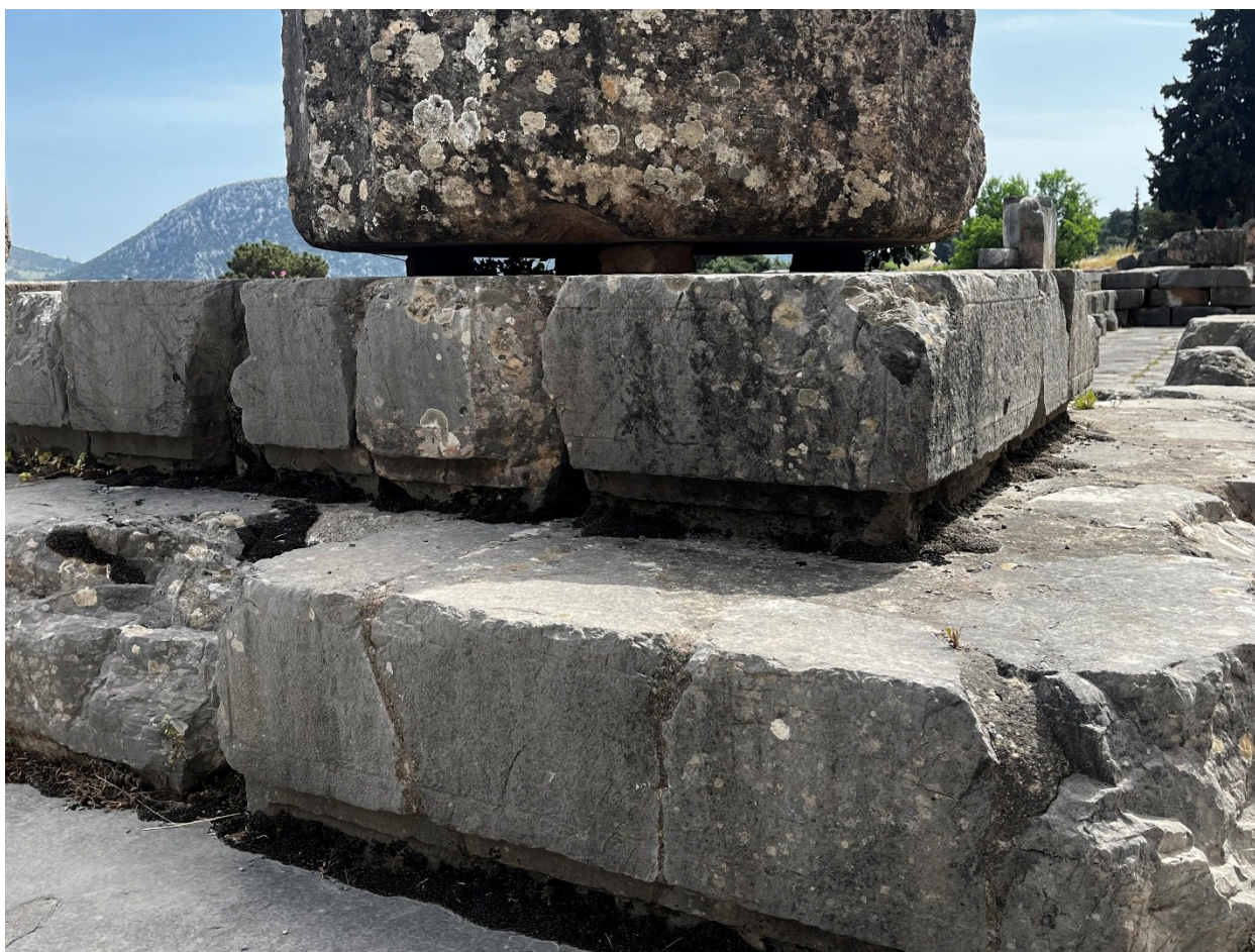
Figure 10. In addition to biological colonization, other deterioration patterns can also be observed on the stone elements, including cracks and localised material loss. Their coexistence within the same architectural area further illustrates that different forms of deterioration may occur simultaneously on the monument.
