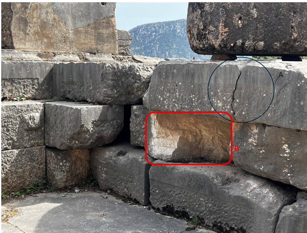
Figure 4. Deterioration patterns observed on stone elements of the crepidoma of the Temple of Apollo: (A) fracture, classified under Crack and Deformation → Crack → Fracture, and (B) fragmentation, classified under Detachment → Fragmentation, according to the ICOMOS–ISCS (2008) terminology (author's photograph, 2026).
