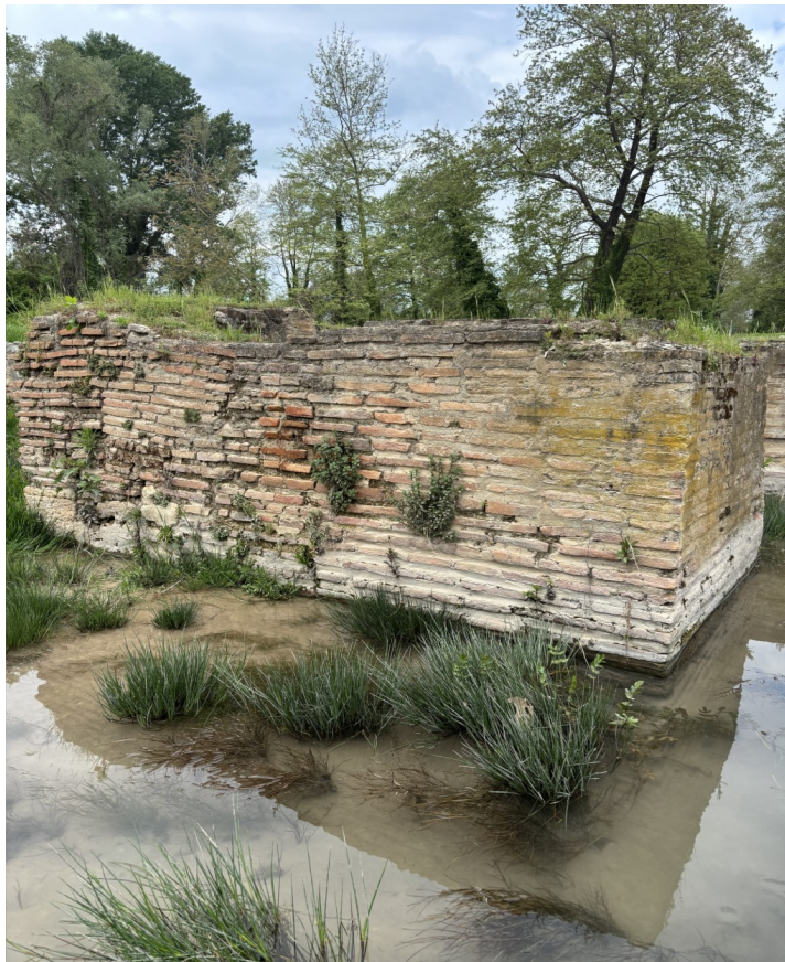
Figure 4.31: Photographic record of the Temple of Isis showing a number of visible signs of pathology: displacement of structural elements, loss of material, biological colonization, cracks, and the presence of vegetation in joints (personal archive).
