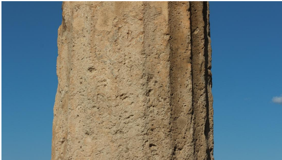
Figure 15. Granular disintegration visible on a column.
