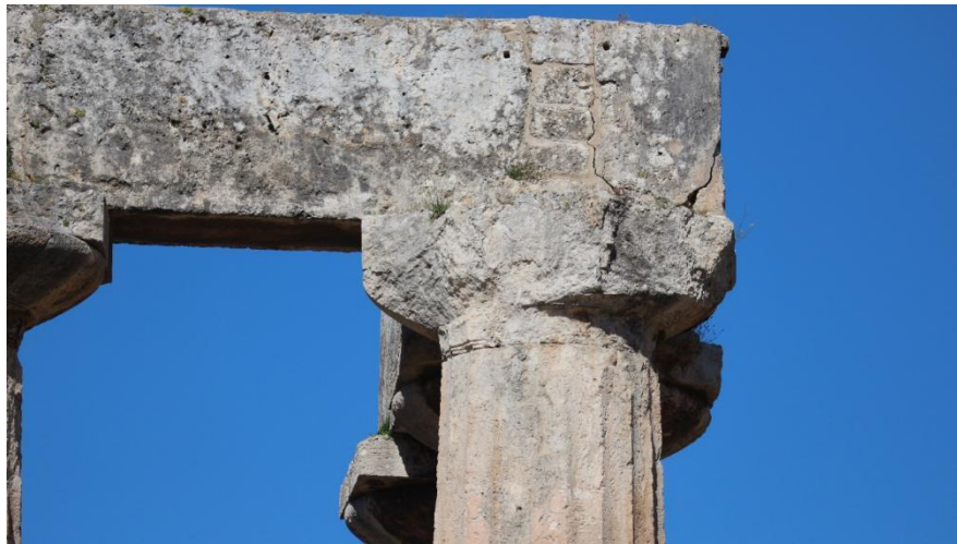
Figure 20. Localized cracking and fracturing affecting an upper structural element.
