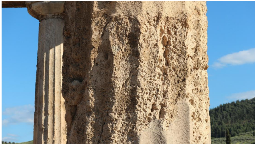
Figure 17. Alveolization on an exposed column surface, showing the development of cavities associated with localized material loss.
