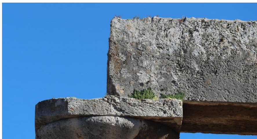
Figure 21. Biological colonization on the stone surface, particularly within joints and moisture-retaining areas.
